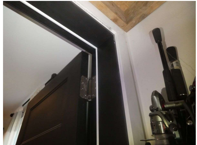
Garage door (man's door)
