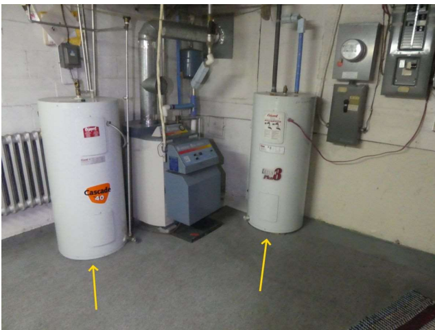
Basement (mechanical room)
