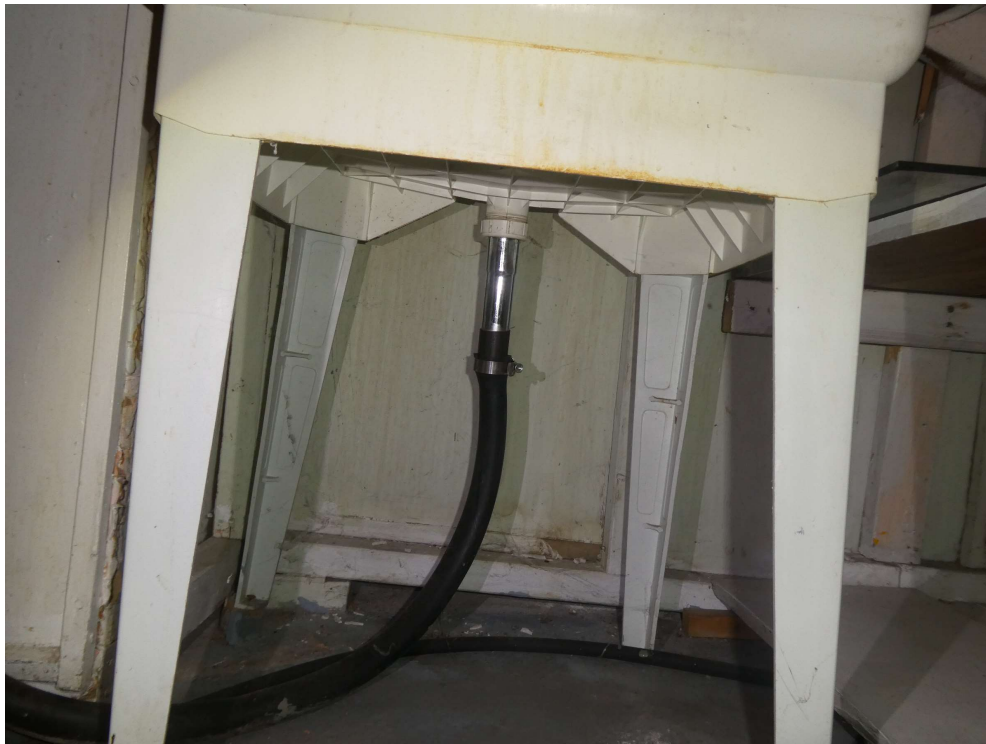
Basement (air exchanger room)
