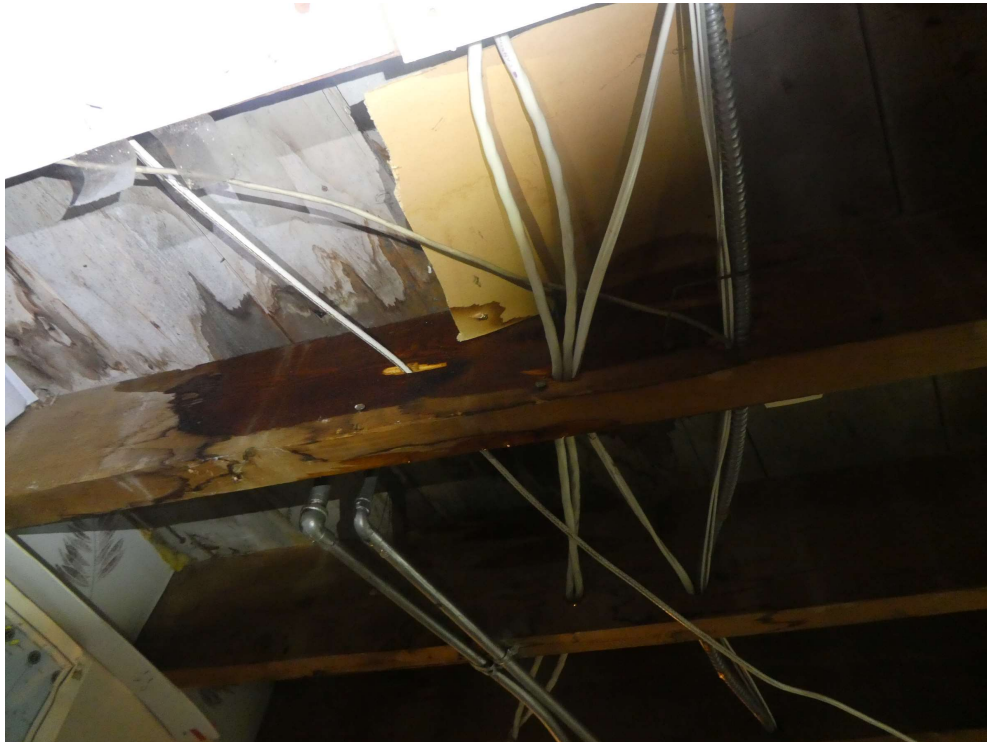
Basement (mechanical room)
