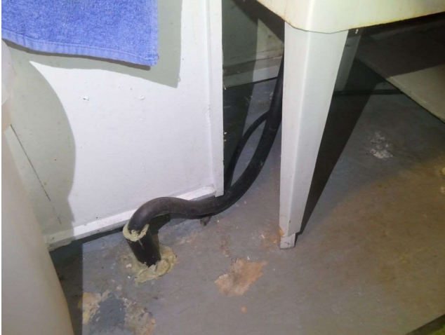
Basement (air exchanger room)
