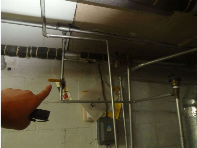
Basement (mechanical room)
