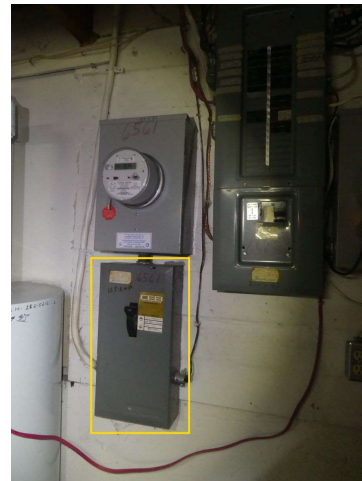
Main disconnect for second floor
