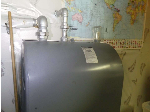
Basement (mechanical room)
