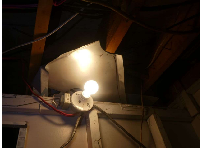
Basement (air exchanger room)
