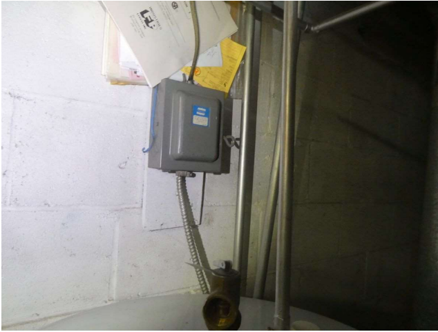
Basement (mechanical room)
