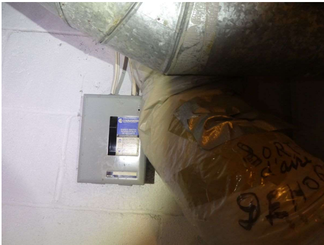
Disconnect for air exchanger
