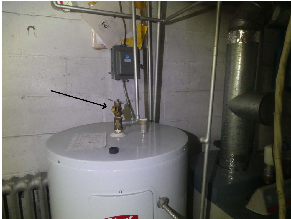
Basement (mechanical room)
