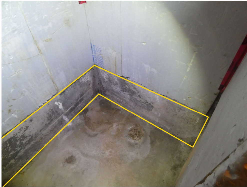
Basement (main water valve closet)
