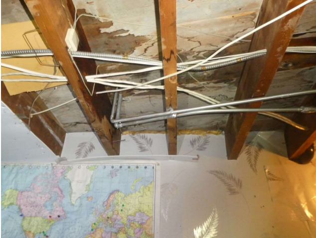
Basement (mechanical room)
