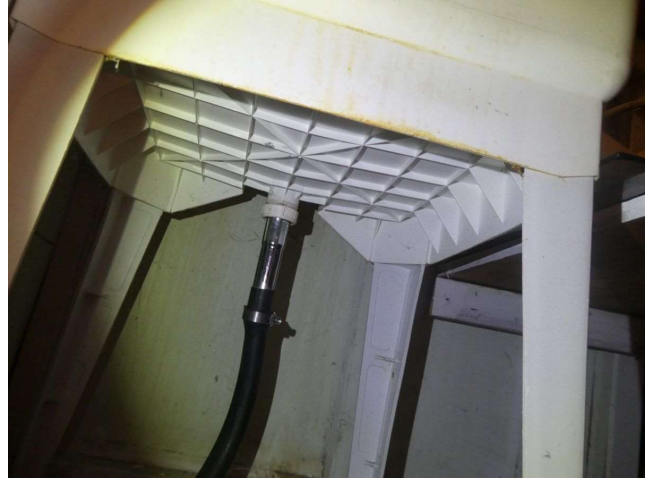
Basement (air exchanger room)
