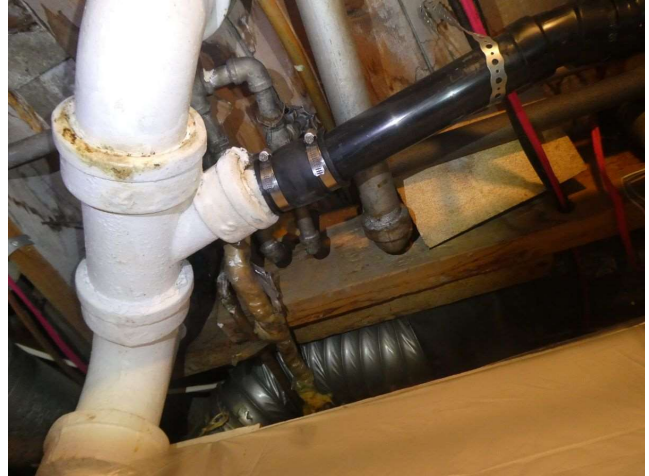
Basement (air exchanger room)
