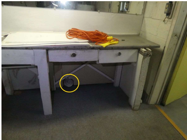
Basement (mechanical room)
