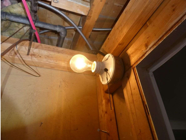
Basement (main valve closet)
