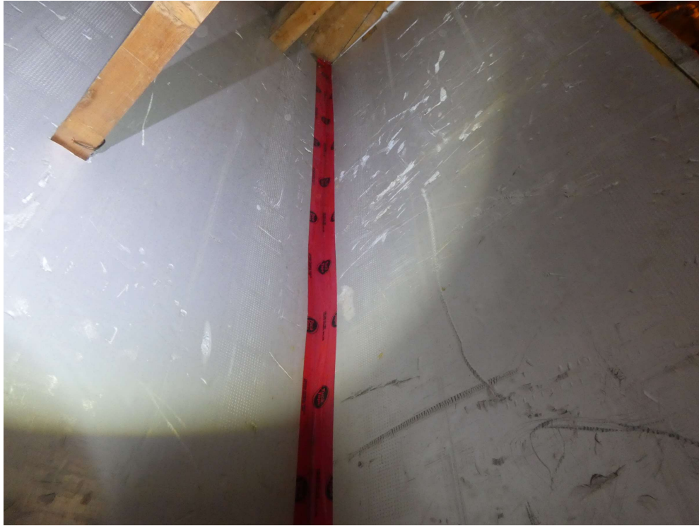
Basement (main valve closet)
